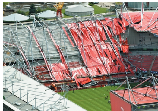
View of stadium damage.
