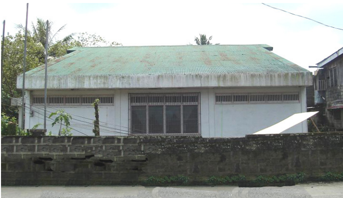
Children's Library building and grounds abut F. Montejo St. BEFORE picture taken a few days into the repair/renovation project. There used to be a huge Talisday tree planted at the front left of center of the Library building which we cut down for safety reasons as the tree was already crowding out the Library building. Also take note of the old faded green roof paint and the weakened CHB fence. Except for limited ventilation the whole front is enclosed making the wide front grounds non-functional.
