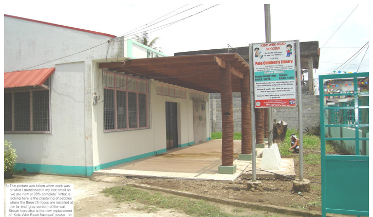
This picture was taken when work was at 98% complete. What is lacking here is the plastering of pebbles where the three logos are installed at the far end (gray portion) of the wall. Shown here is the new replacement of "Kids Who Read Succeed" sign, new porch supported by beams, new windows and the fully-working sliding tinted-glass door
