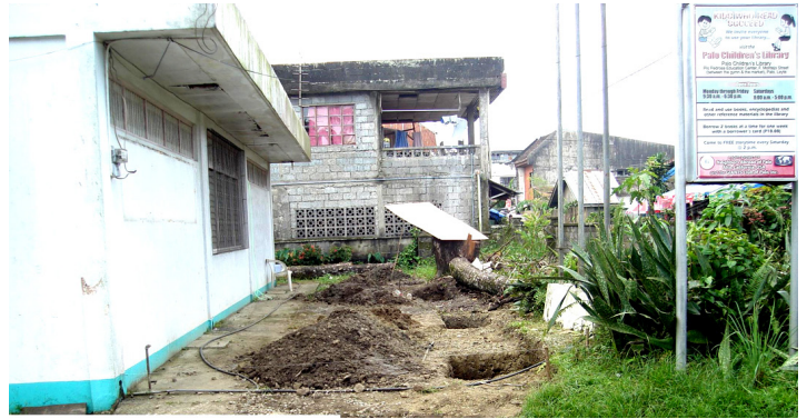
The initial work on the ground for the repair/renovation of the childrens library has just started. The weakened low CB fence at the far end will be demolished and replaced with a new reinforced much higher CHB fence. The trunk of the Talisday tree we cut down (lying on the ground) was sliced up and made into trellis to support our polycarbonate cover to save cost on lumber. Please take note of the faded surface of our "Kids who Read Succeed" poster and the failing metal on its underside with its electrical wiring inside damaged and no longer working. Except for the iron posts, we have it all replaced.
